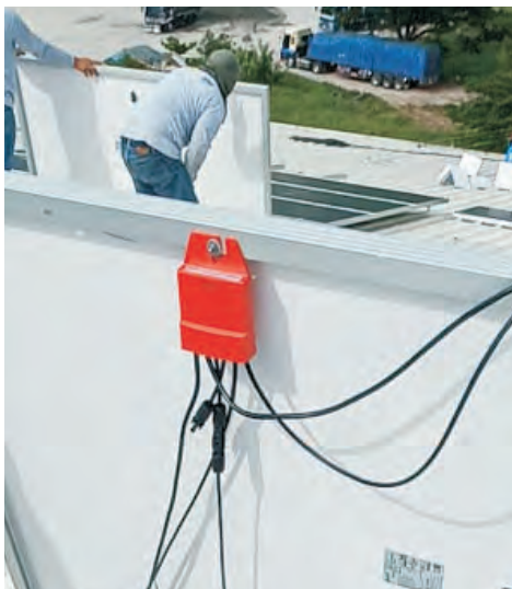
CASE STUDY: Bulacan, Philippines with 200kwp solar installation.
