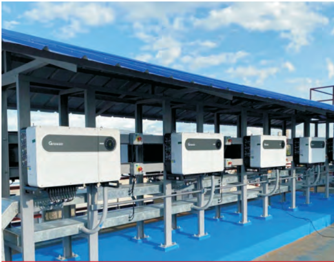
CASE STUDY: Philippines with 1.2MW solar installation.
