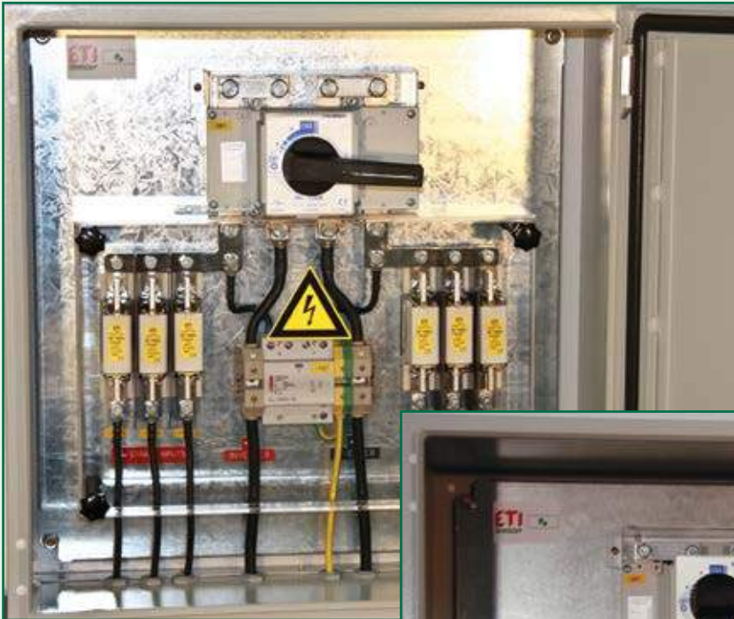
DC junction box (NH gPV fuses)
