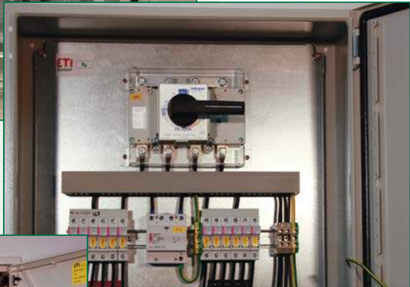
DC junction box (CH gPV fuses)
