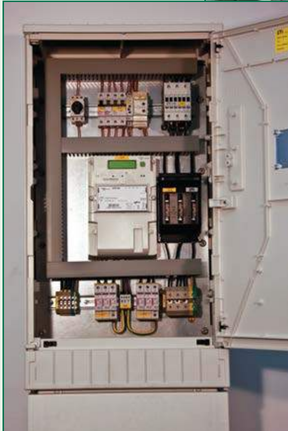
Meter distribution cabinet
