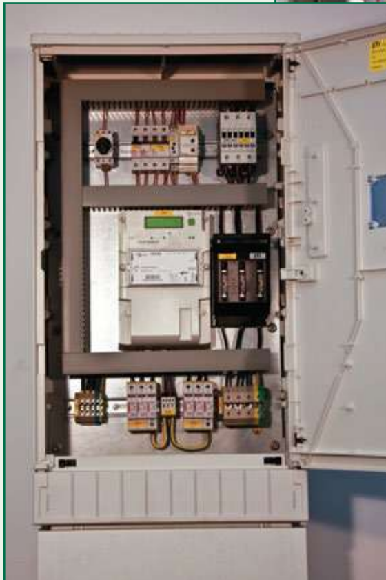
Meter distribution cabinet
