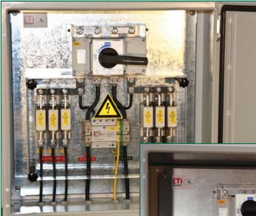
DC junction box (NH gPV fuses)
