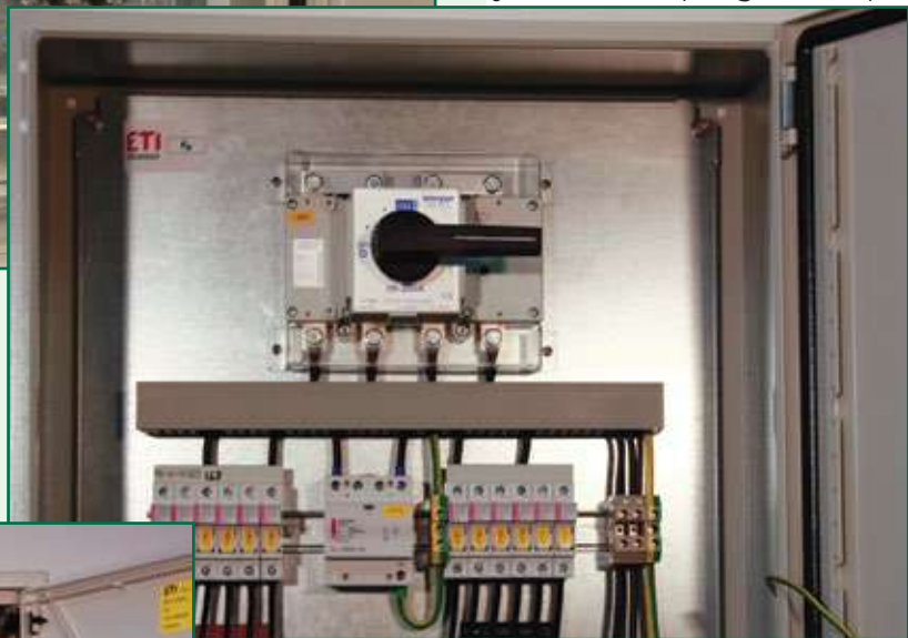
DC junction box (CH gPV fuses)
